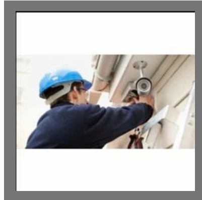
CCTV Camera & DVR AMC Service
